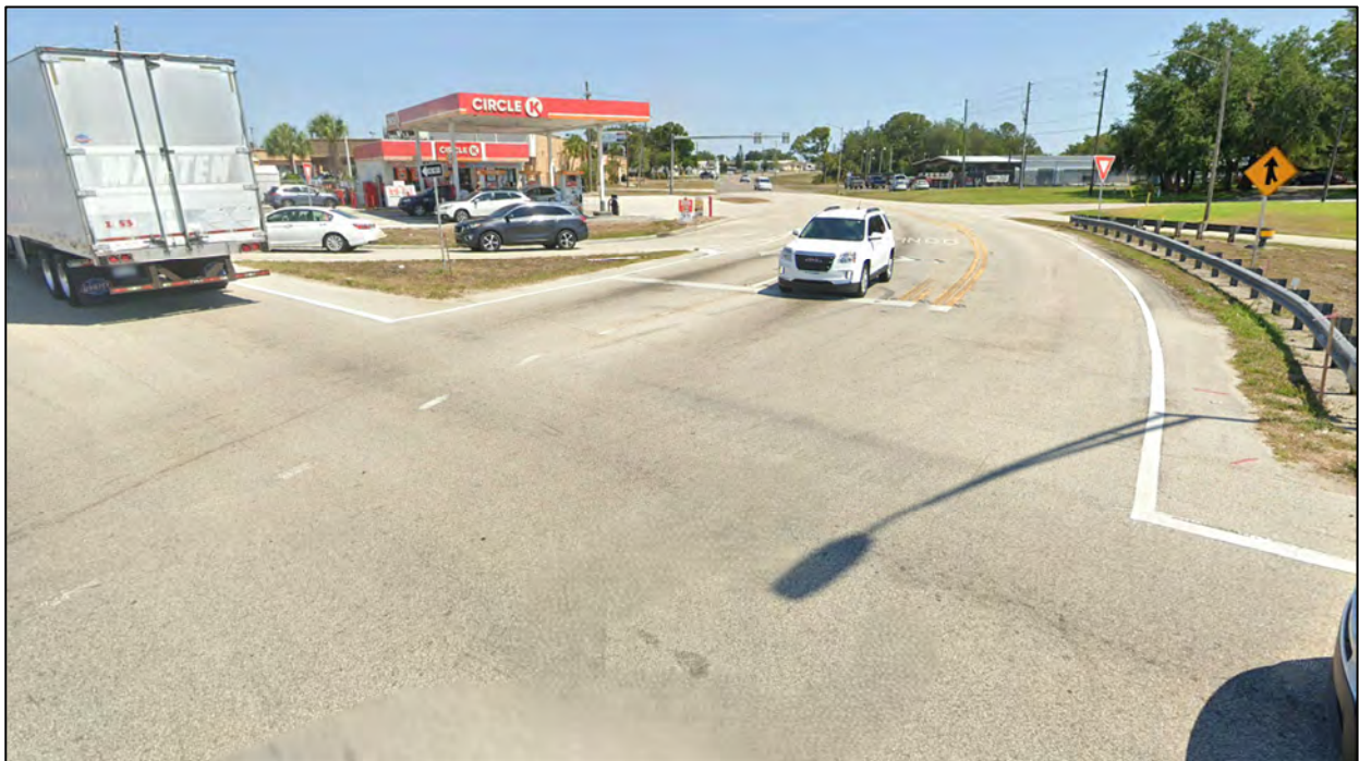
Figure 14: Existing Conditions of the segment of Sebring Drive
